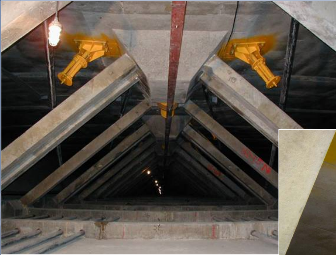
Stay Cable Dampners
